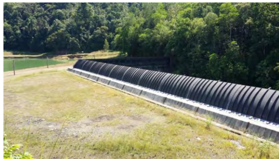
Figure C.11: Pneumatically Actuated Gates (Obermeyer Spillway) at Babagon Dam provided by Jabatan Air Sabah)
