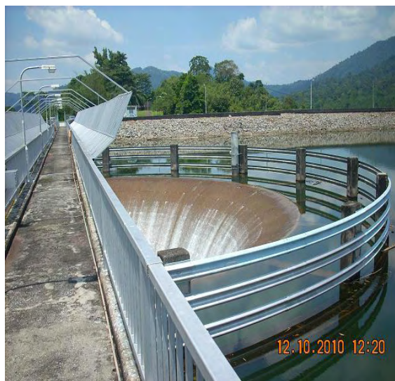
Figure C.14: Morning Glory Spillway – Sungai Langat Dam (provided by Pengurusan Air Selangor Sdn Bhd)
