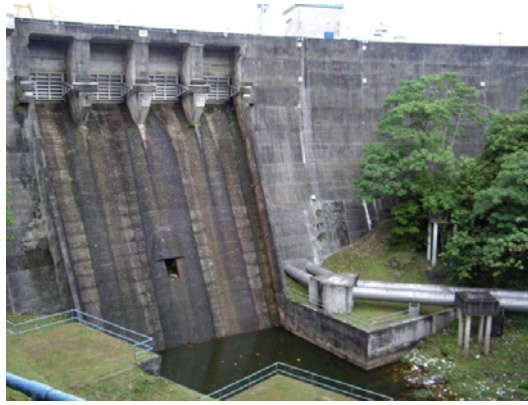
Figure C.10: Vertical Lift Wheel Gate at Klang Gates Dam (provided by Lembaga Urus Air Selangor)
