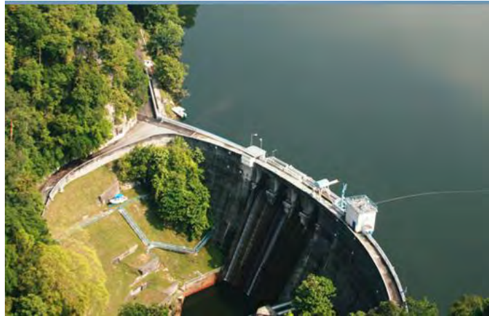
Figure C.6: Concrete Gravity Dam – Klang Gates Dam (provided by Puncak Niaga (M) Sdn Bhd)
